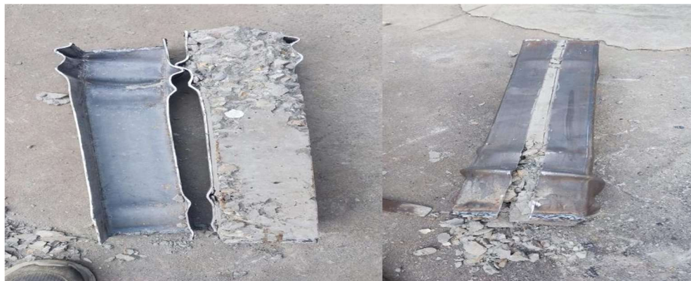
Fig. 6. Failure modes observed in SFFSST columns
